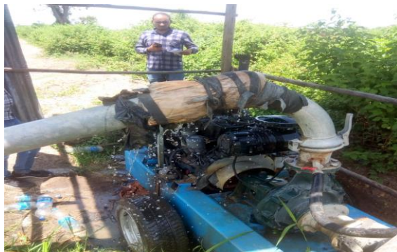
Fig 24:- Some problem observation on unfitting of delivery water pipe during data collection
