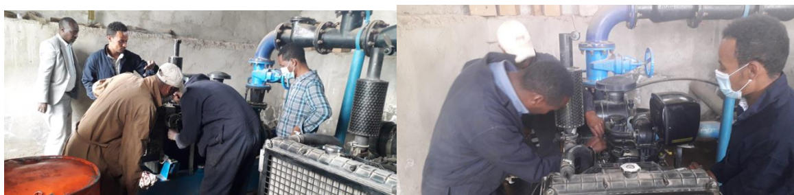
Figure 32. Shows during pump maintenance takes place
