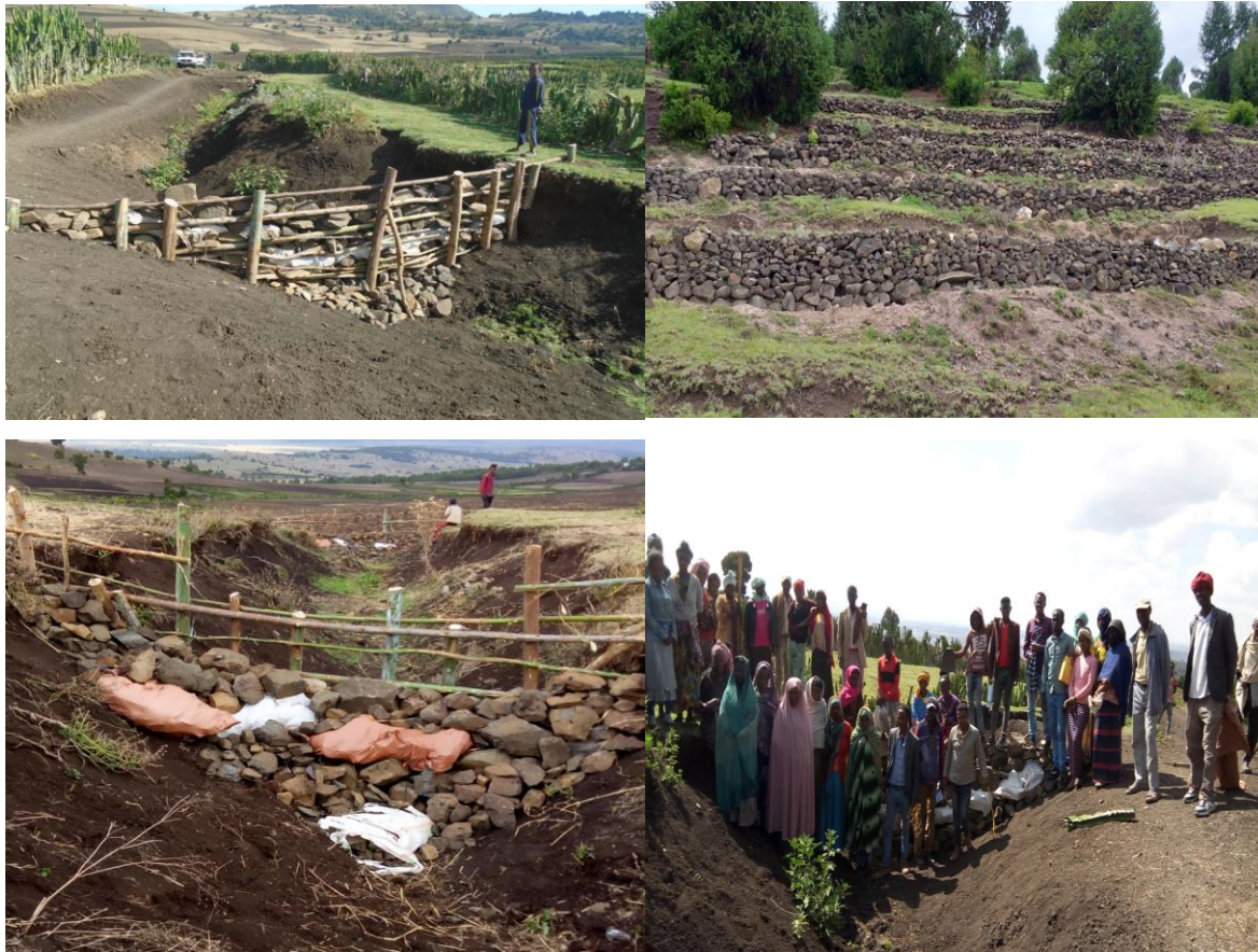
Figure 3. Picture during community based participation in implementing soil and water conservation structures in Ilasa watershed.
